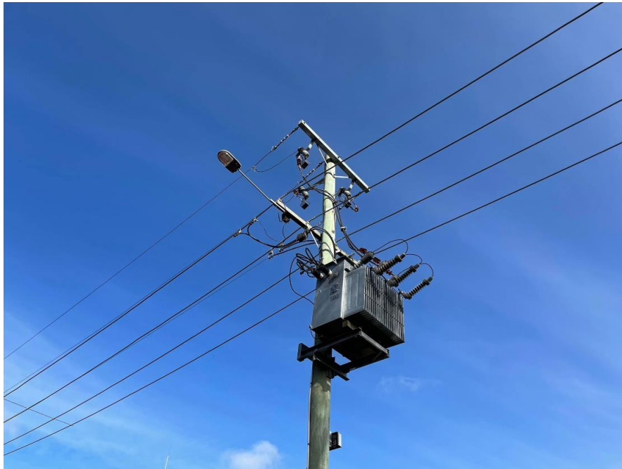
Figure 13: 500 kVA Market Street Transformer
